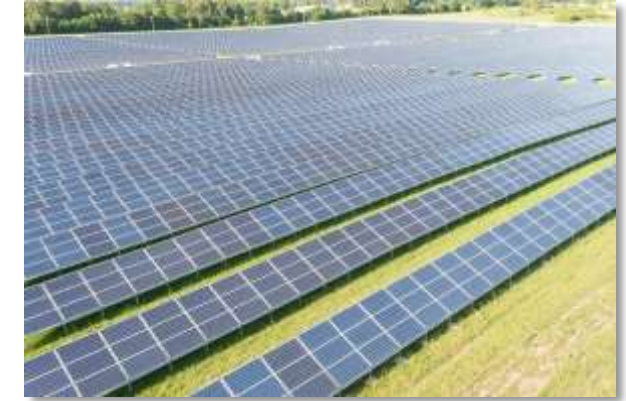
Ground mounted Solar Park
