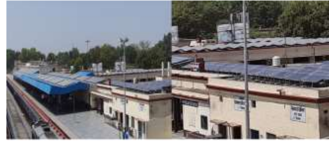
Installed 265 KWp at Faizabad Railway station
